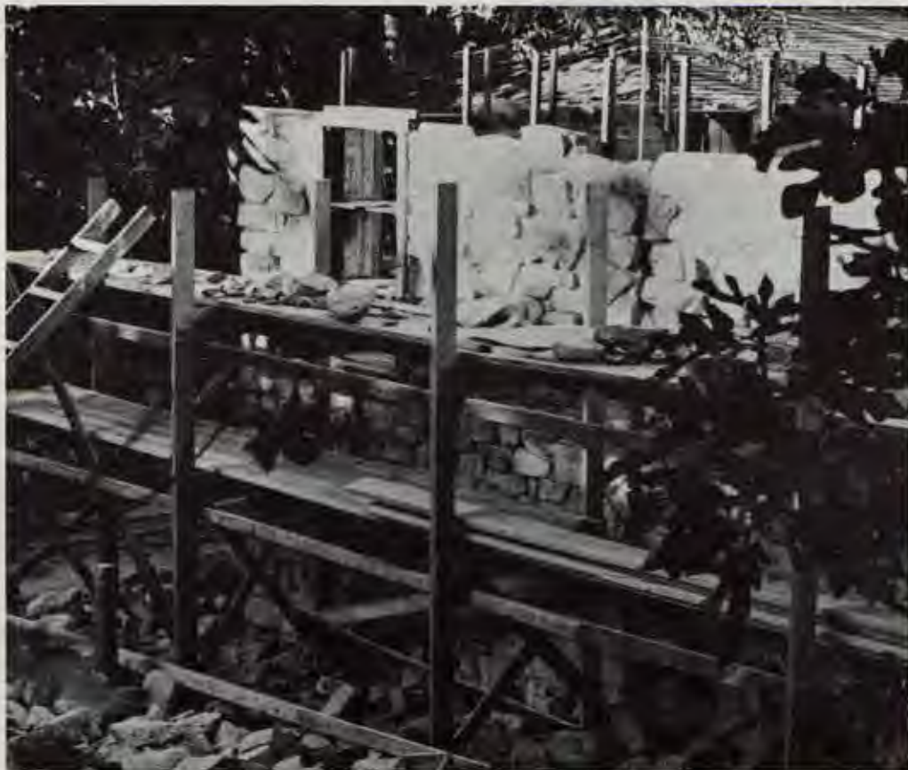
In November the masons at Tassajara completed the stone walls of the new kitchen. By the New Year the carpenters should have the roof on.
