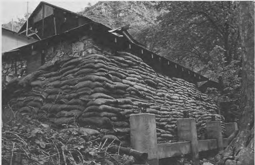
Flood protection for the basement food storage area.
