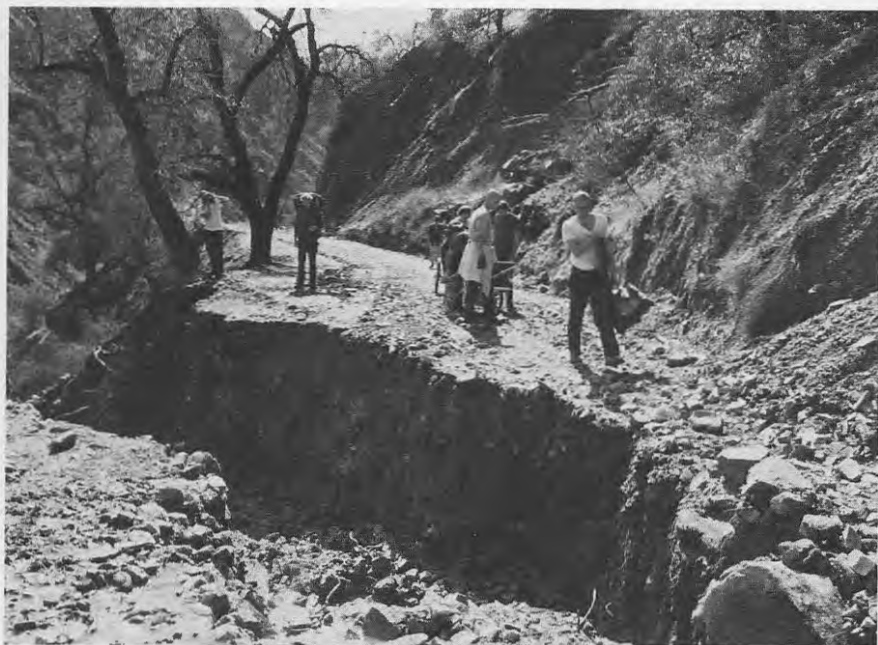
One of several spots where the Tassajara roadbed washed completely away.
