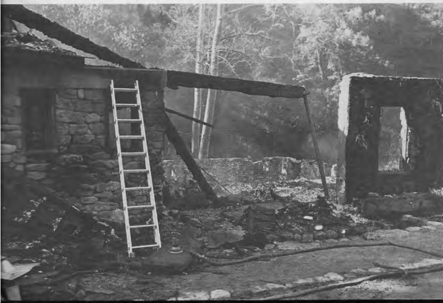
The ladder stands to the left of what used to be the Zendo entryway.
