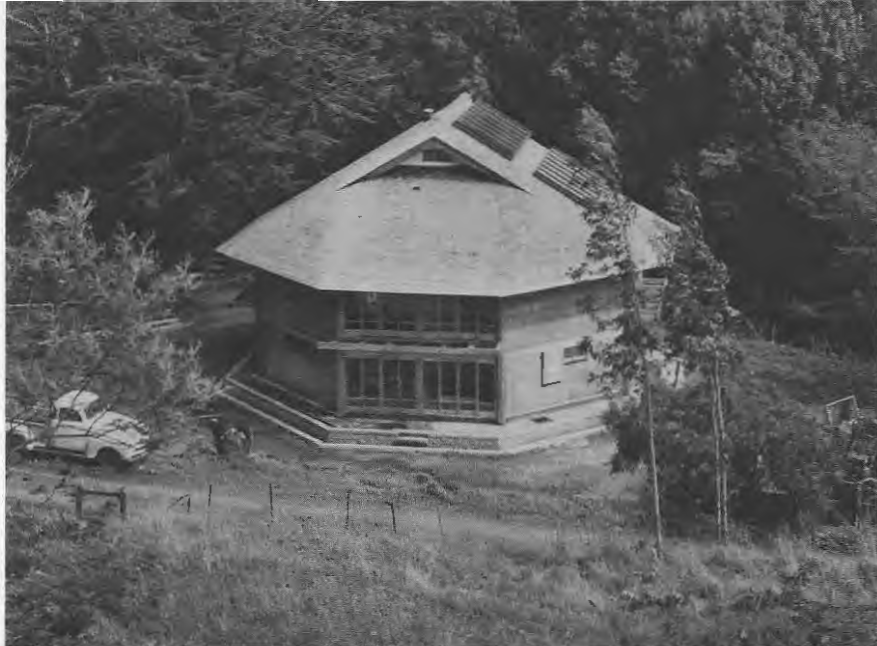
Lindisfarne Hall near completion. It was designed by Green Gulch Head Carpenter Paul Discoe, with the help of architect Sim Van der Ryn. The octagonal plan echoes the lodge plan of the Miwok Indians, our predecessors in the Green Gulch valley.
