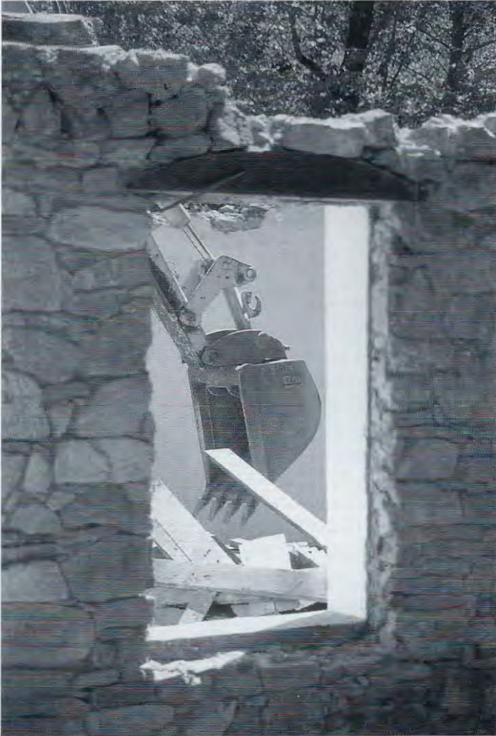
The 100-year-old Tassajara stone dining room was renovated during the fall, winter and spring of 1997-98. It will be completed in time for the opening of the Tassajara guest season on May 8.
