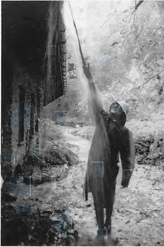
Work leader Kosho McCall cleans out the Stone Rooms rain gutters at Tassajara.
